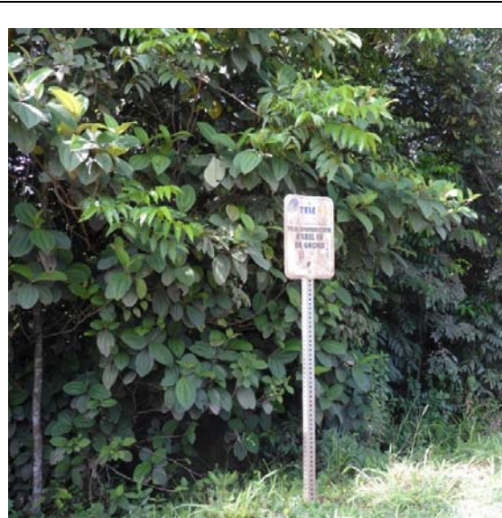
Photo 10: Telesur underground cable along the Brownsweg
