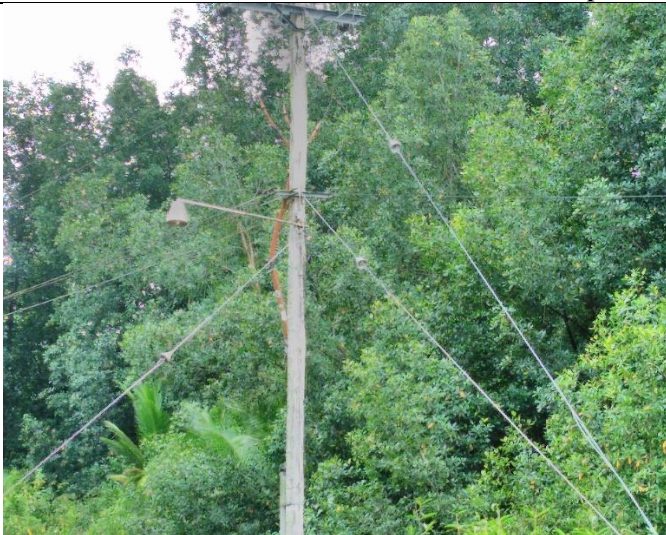
Location at current 12 kV single-circuit line (red cable) at Plantation Kroonenburg
